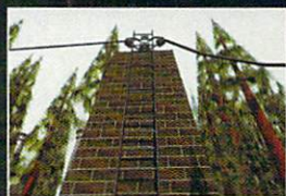
Ah ha! A power trip-switch. Now then, maybe if I throw it, the power will be re-connected!
